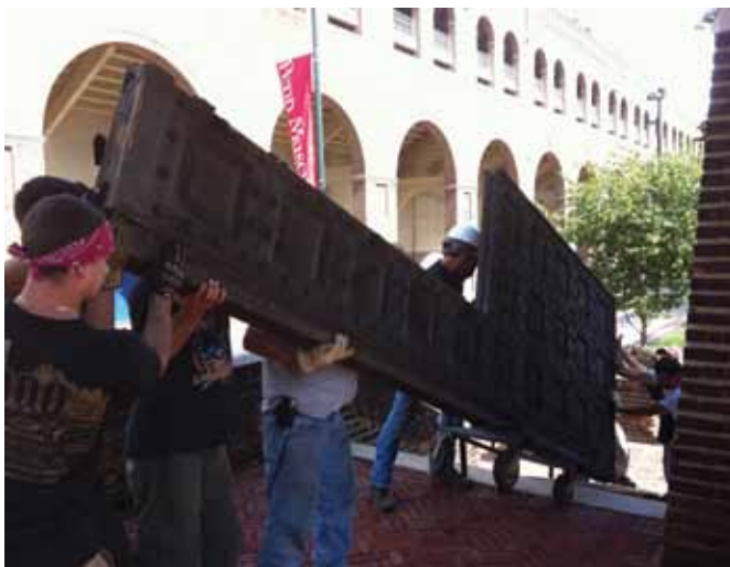
One of the oversized doors at the Upper Main Entrance was removed for renovation in August 2011.
