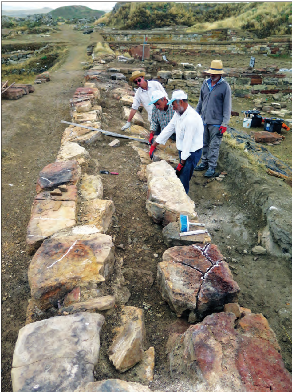
Figure 4: Conserving the back wall of Terrace Building Unit 6, which was badly damaged by the fire of ca. 800 BCE. Photo by Brian Rose
