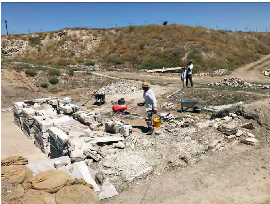
Figure 5: The conservation of Megaron 3, looking west. The disintegrated state of the wall is visible at right; the new stone encasement is at left. Photo by Elisa Del Bono.
