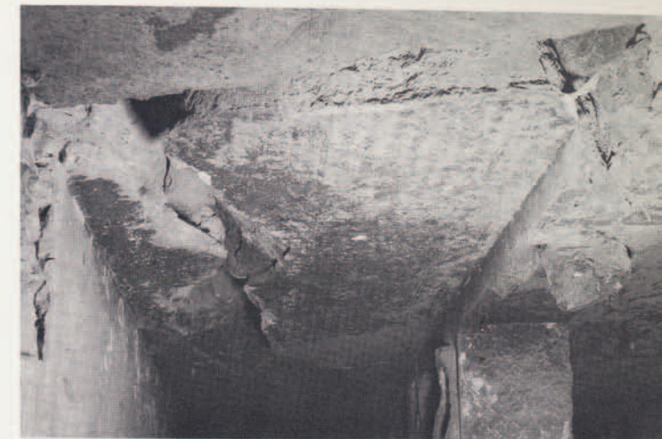
Large cracks in limestone ceiling of broad-hall of tomb of Nebwenenef. Lower right, upper parts of two Osirid pillars, one still standing, the other destroyed.
