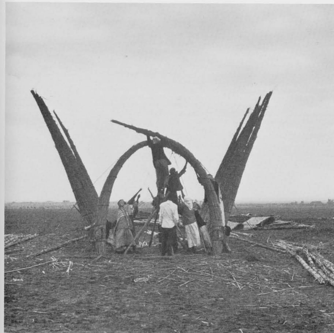
3 Building a mudhit . From the bundles of reeds planted at the sides of the structure, individual reeds are bent to form the domed roof of this "quonset"-type house. The whole will be covered with reed matting.
