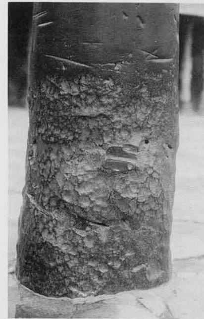
5 The pillar, which was erected only about 1600 years ago, shows serious rust pitting at its base. (Photograph by Robert Raymond)
