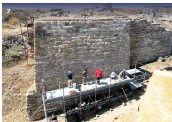
(1) Conservation at the citadel's East Gate (9th century BCE), looking west. Photo by Brian Rose. (2) Conservation of the East Gate's South Bastion, looking south (9th century BCE). Photo by Brian Rose.
